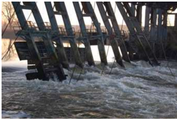
Figure 1.2: weir Grave after ship collision [46]
